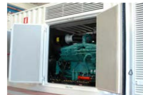
Container 60/65 dbA - 40" HC 1400 kVA Cummins
